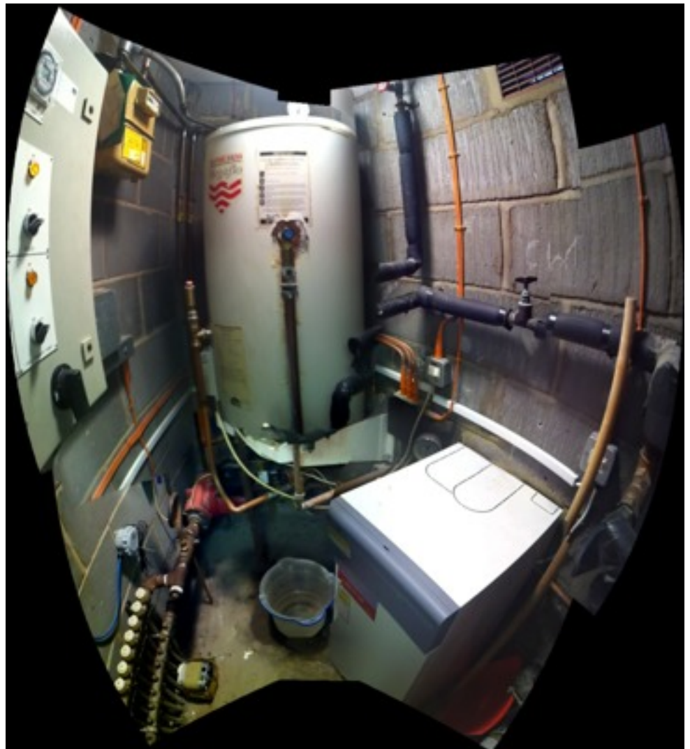
Inside the boiler room shows the Megaflo which even though it is only 5 years old can no longer function due to limescale!
