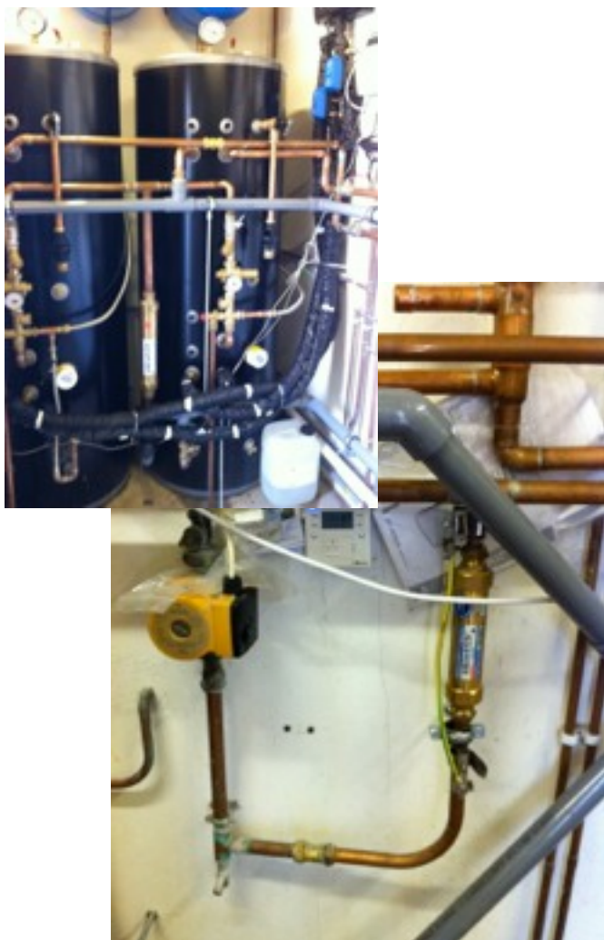
The AQUABION®s installed on the mains and on the Secondary Return
