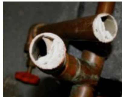
These pipes show the extent of the limescaling problem on this holiday site
