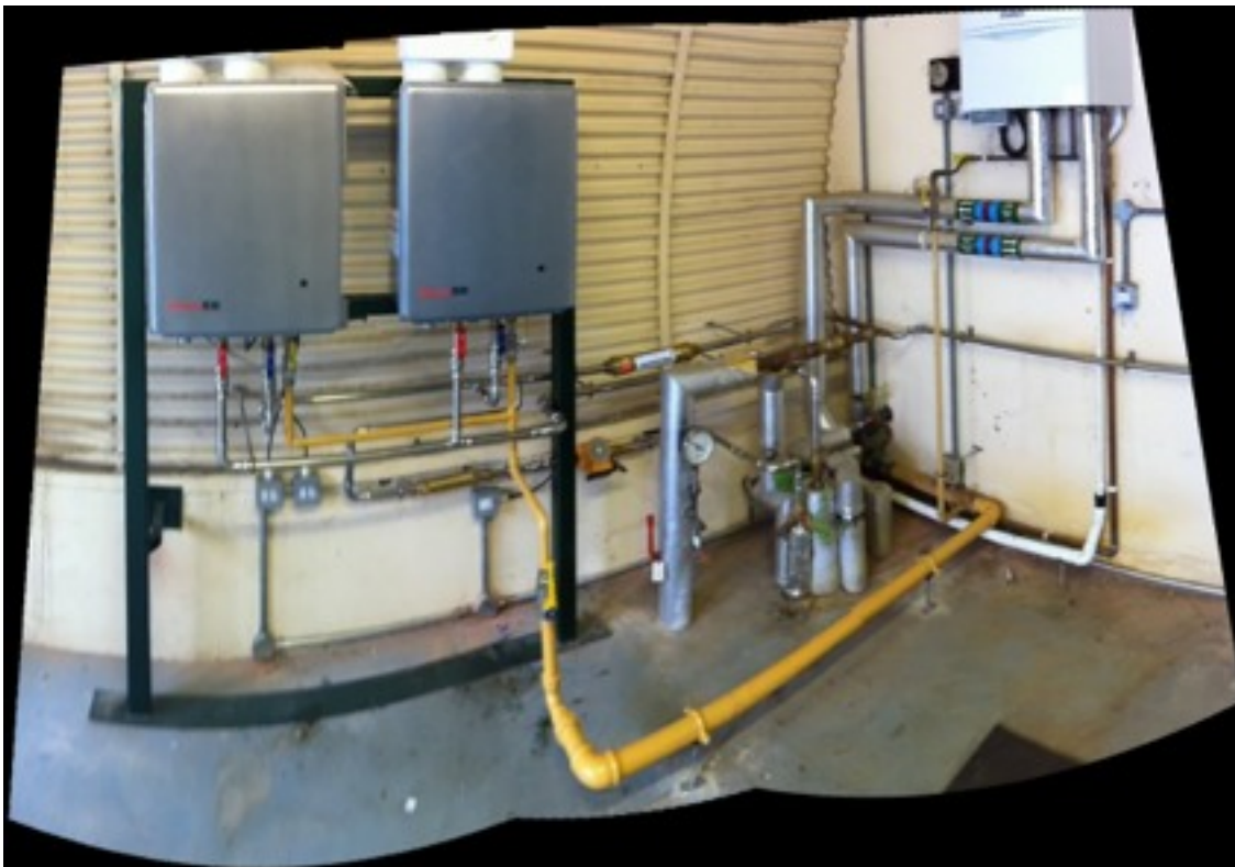
One of the successful installations for Landmarc on behalf of the MOD
