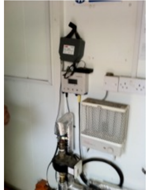
Other water treatment systems did not stop the Rinnai warm water heater from scaling up
