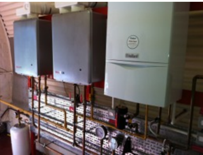
The Rinnai hot water heaters and boiler for the central heating system
